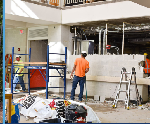
Taking down the concrete wall that separated the kitchen from the dining hall – January 2021
