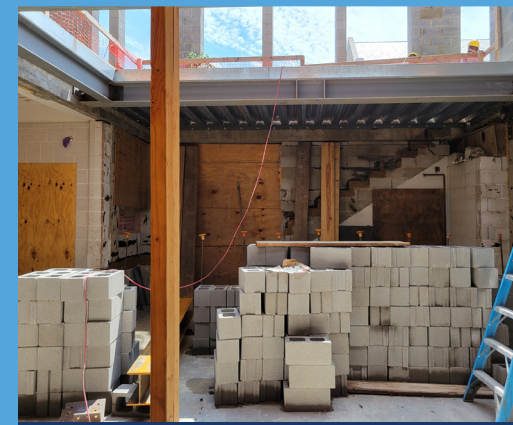
Steel and concrete going in to enclose the lower level courtyard – July 2021
