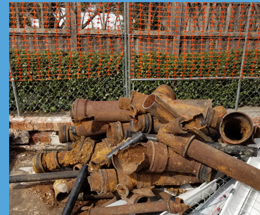
Plumbing and ceiling debris from the kitchen – February 2021
